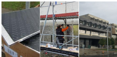
Vacuum Insulation Panel (VIP) 3cm thick and 110x700 mm, its placing and UPV/EHU building demo site after Super insulated façade installation
