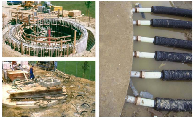
Fig. 39: realization of hybrid STES in Attenkirchen, Germany (source: ZAE Bayern and Solites)
