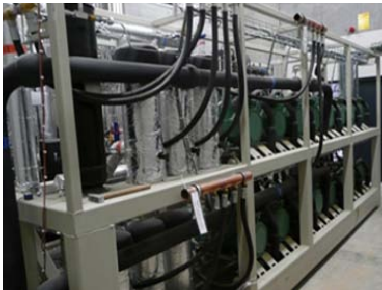
Fig. 50: One example of the successful integration of a heat pump is the pilot project Sunstore 4 in Marstal, Denmark (source: solites)
