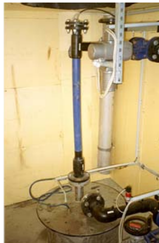
Fig. 35: Wellhead in the well house (source: solites)
