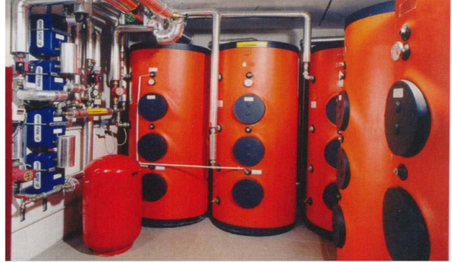
Fig. 41: “Collection” of buffer storages in retrofitting application where a larger storage could not pass the way into the technical room (source: Solites)
