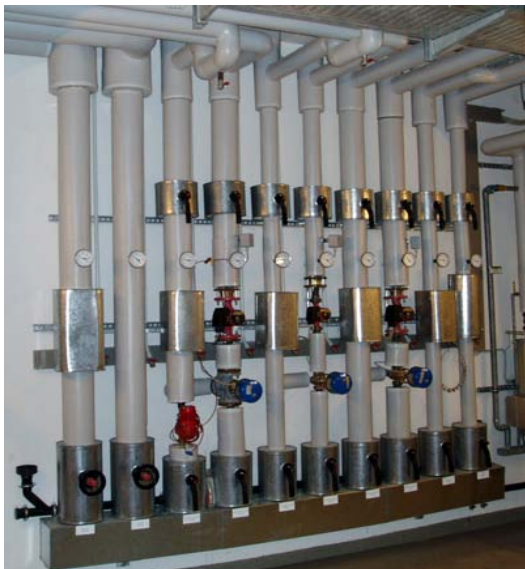
Fig. 49: The illustrated example of a heat distributor as part of the heat supply shows the interplay of various system components (source: solites)
