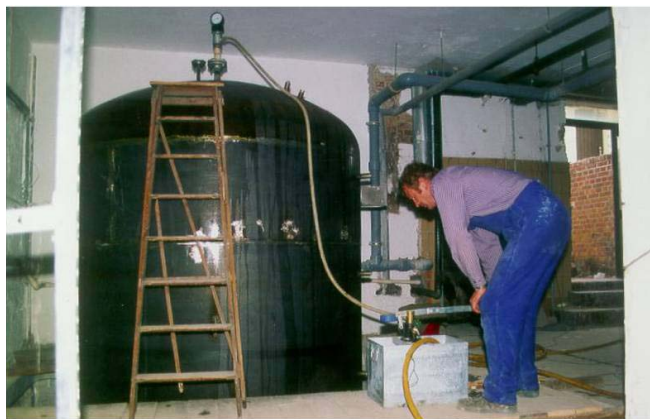
Fig. 42: Integration of a large buffer storage in retrofitting application by using two floors and removing the floor in between (source: Solites)
