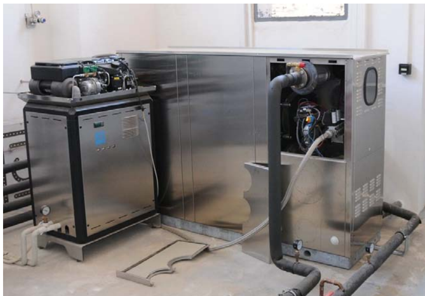
Figure 3. Prototype H 2 burner and condensing boiler.
