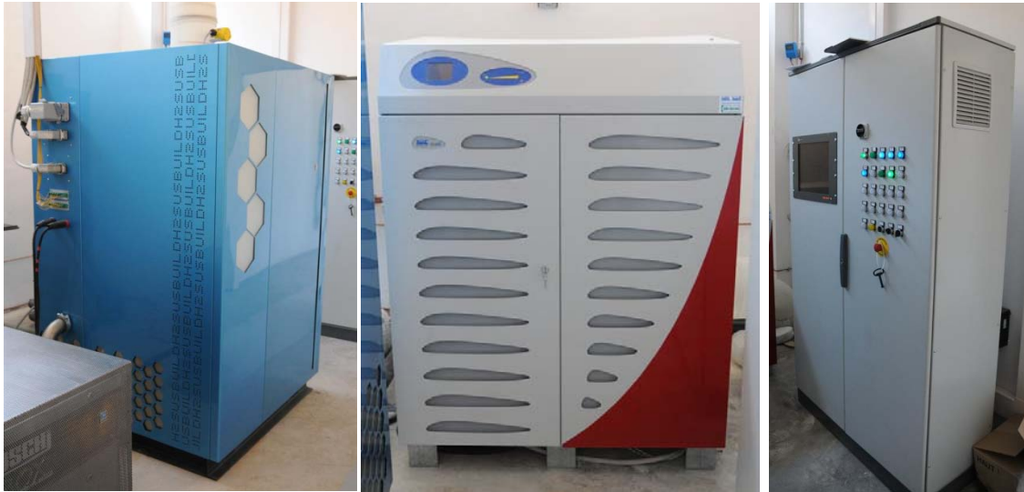
Figure 2. From left to right: a) Micro-CHP FC, b) inverter and c) Control cabinet.
