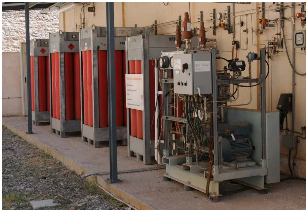
Figure 5. New pressure cylinder stacks for the storage area.
